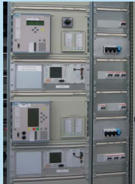
Twin transformers (REGSys voltage regulation systems with REG-D voltage regulator and REG-PE protocol card)
