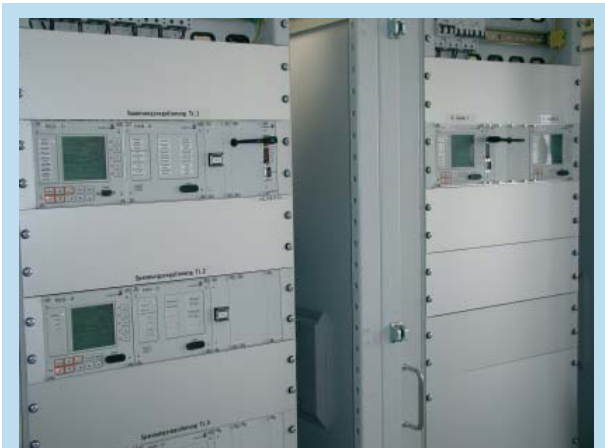
Stadtwerke Trier GmbH, Werner-Siemens-Str. substation with IEC 61850 connectivities. Three REGSys voltage regulation systems (left) with REG-D voltage regulator, PAN-D monitoring unit, REG-FR tap changer interface and two REG-DP Petersen coil regulators (right), each linked to the control systems via an IEC 61850 REG-PE protocol card.
