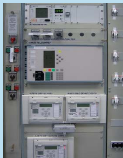
Single transformer (REGSys voltage regulation systems with REG-D voltage regulator and PAN-A1 monitoring unit - RWE version)
