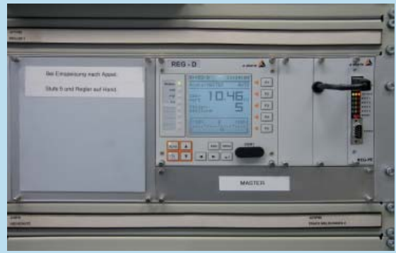
RWE Westfalen-Weser-Ems Netzservice GmbH / Dortmund / Germany, Lüdinghausen substation with different IEC 61850 connectivities
