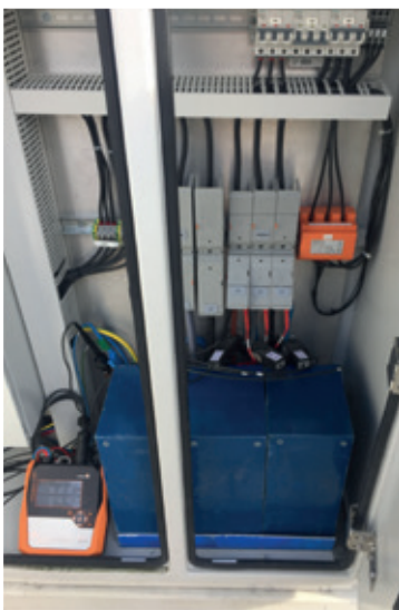
Figure 3: Measurements with PQ-Box 150
